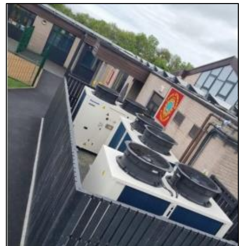
Figure 3 - Heat Pumps at Ysgol Kingsland
