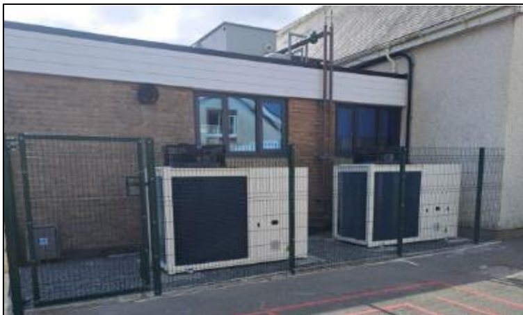
Figure 2 - Heat Pumps at Ysgol Rhosneigr
